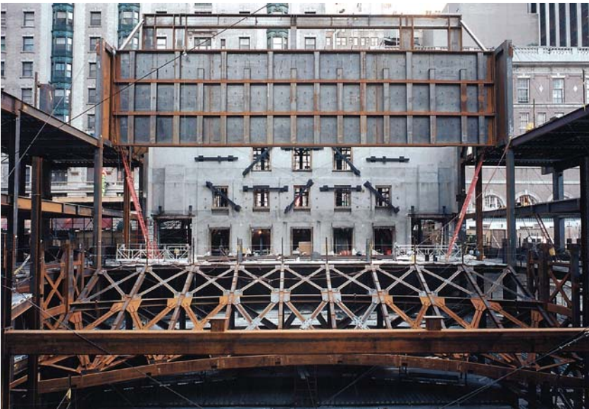
Photo shows the back of the façade of Henry Miller's Theatre. On this side of the façade, the theater's steel structure takes shape. The curved, 85-foot steel beam will support the mezzanine. Photo courtesy Bernstein Associates.
