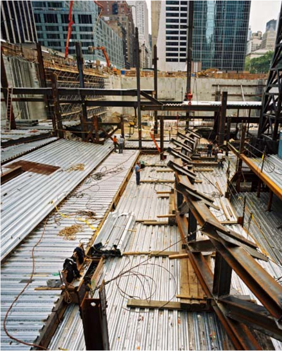
Construction of Henry Miller's Theatre. An 85-foot-long curved steel beam supports the mezzanine. Photo courtesy Bernstein Associates.
